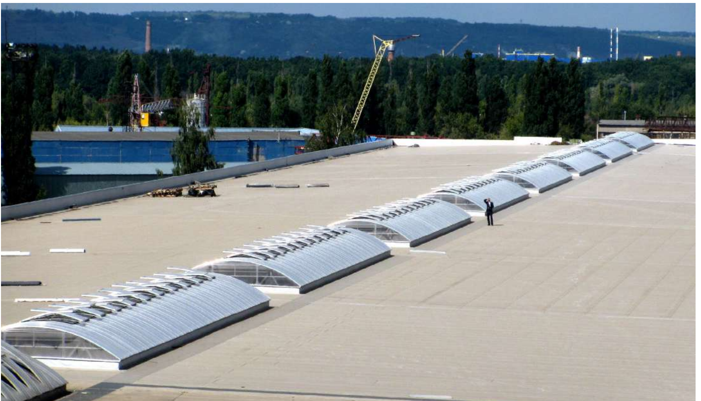
Gable ridge flat skylights 6,14 x 48,0 m with smoke extraction and ventilation doors, 20 items (total area of the skylights is 2 650 sq.m.)
