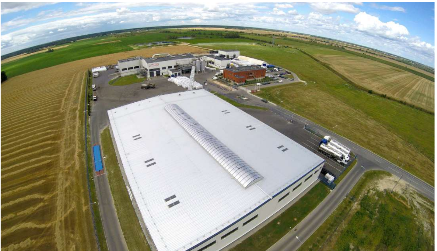
Gable ridge flat skylight 6,0 x 53,8 m with smoke extraction and ventilation doors
